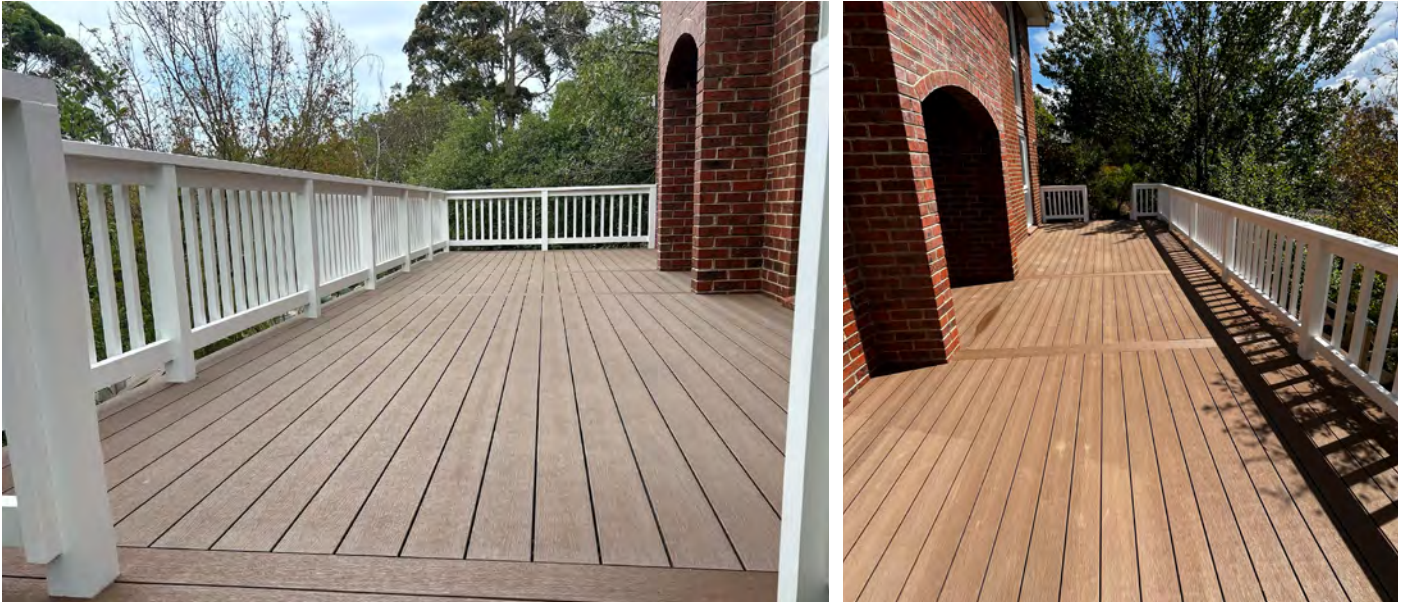
The Sustainable Decking Co. installed this stunning Everdeck project in Nutmeg Brown.
